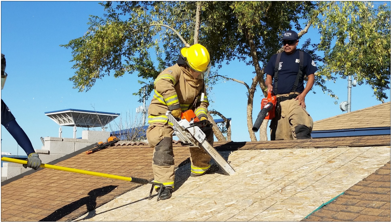
Firefighter Apprentice trainee Jessica Lewis learns how to ventilate a building during a fire training drill. For more on Jessica’s story, see page 17. (Photo: Gila River Employment & Training Department)
