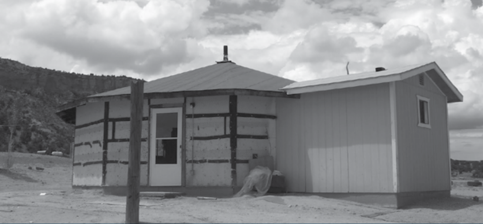
Many tribal homes are still not up to modern safety standards like this image taken on the Navajo Nation in Arizona. Photo credit: Department of the Interior
